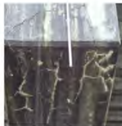
Discharged ASR gel through cracks: macroscopic motion
