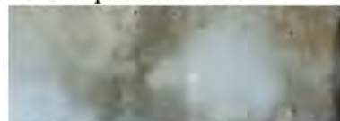
Crack closure with expelled water
