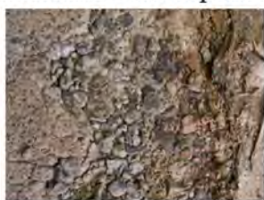
Disintegrated concrete after fatigue + stagnant water
