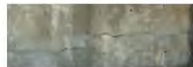
Crack open in water
