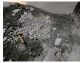
Degradation of concrete slabs
