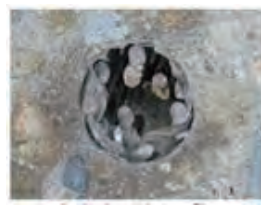
Ducts unfilled with grout
