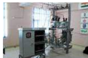
Advanced Metering Infrastructure in Panipat, India.
