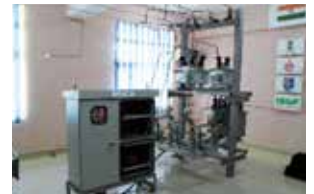
Advanced Metering Infrastructure in Panipat, India.
