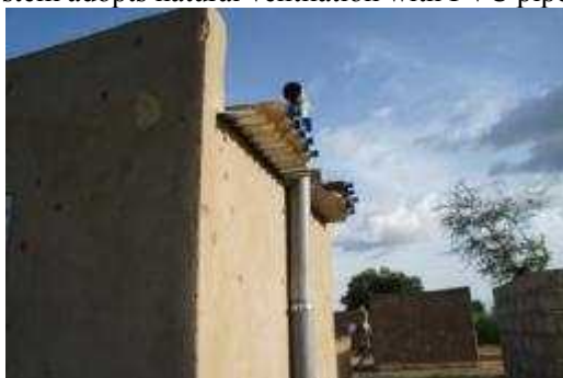
Figure vi) Outlet of ventilation tube
