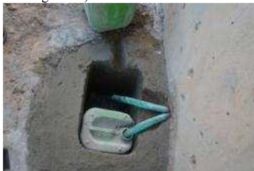
Figure v) Outlet and tank for urine collection
