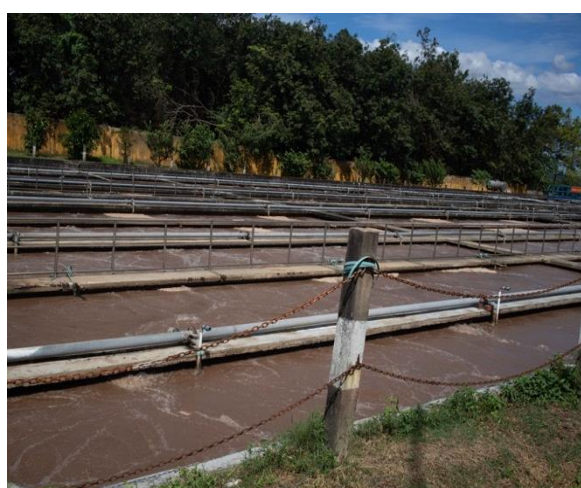
Fig. 6 Industrial wastewater treatment system.
