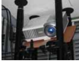
Fig. 7. Projector on Ceiling
