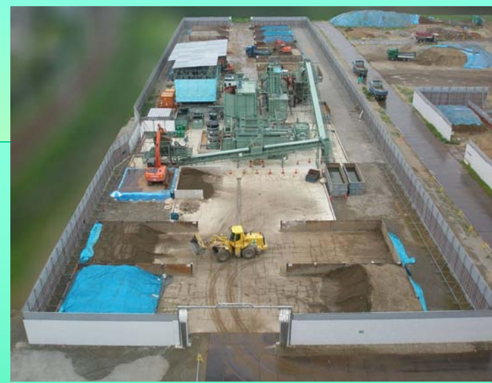
View of on site treatment. (offered by Takenaka Corp. and Takenaka Civil Eng.& Const. Co., Ltd.)
