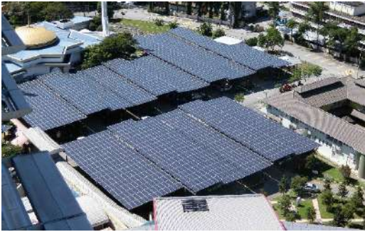
Solar panels above the parking
